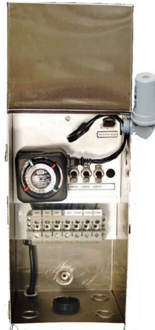
Figure 3 – 24 hour clock timer and photocell installation
