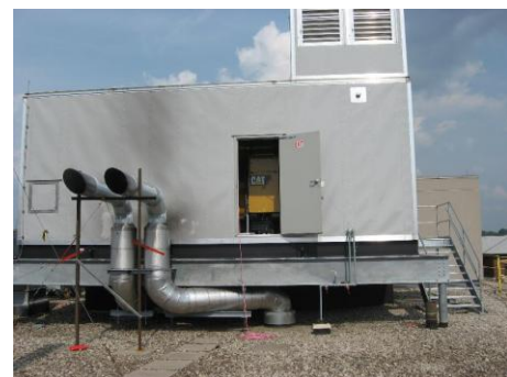
Fig 7a. Magee Rooftop Installation.
